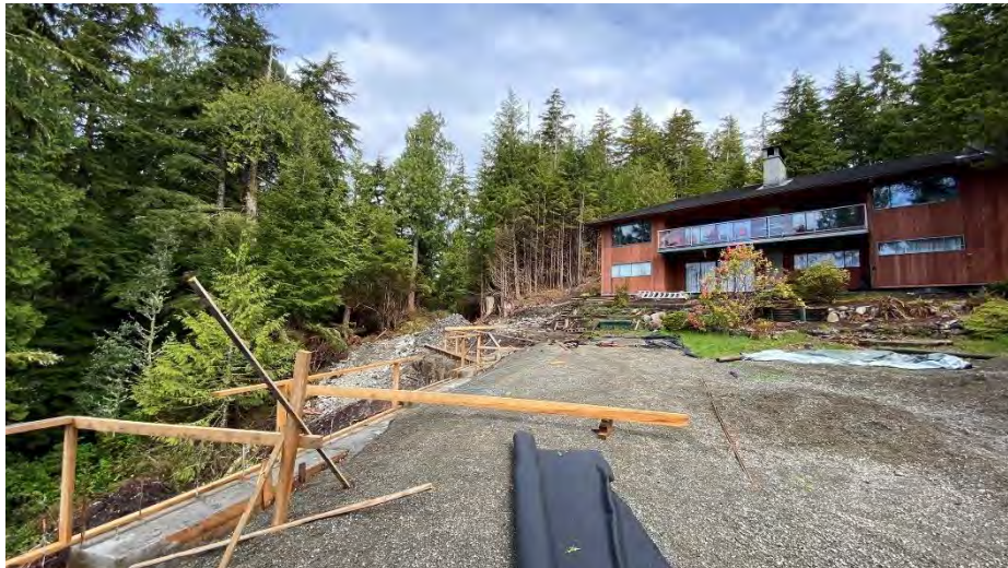
Photo 4. Looking north at house site within Lot B (retaining wall construction in the foreground).
